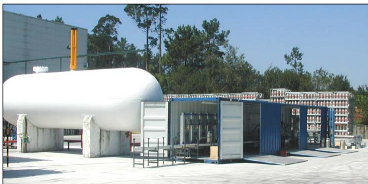
Complete container filling plant with storage tank
